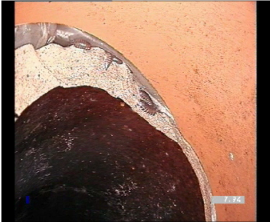
Photo: 4_4A, VCR No.: 010208_1 24FT, Vermin Other, quantity: 2 cm, within 8 inches of joint: NO / cannot be determined
