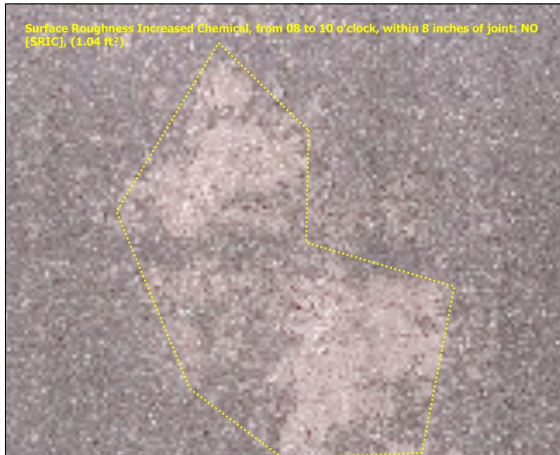
Photo: 7_11A, Media No.: 010208_1 244.14FT, Surface Roughness Increased Chemical, from 08 to 10 o'clock, within 8 inches of joint: NO
