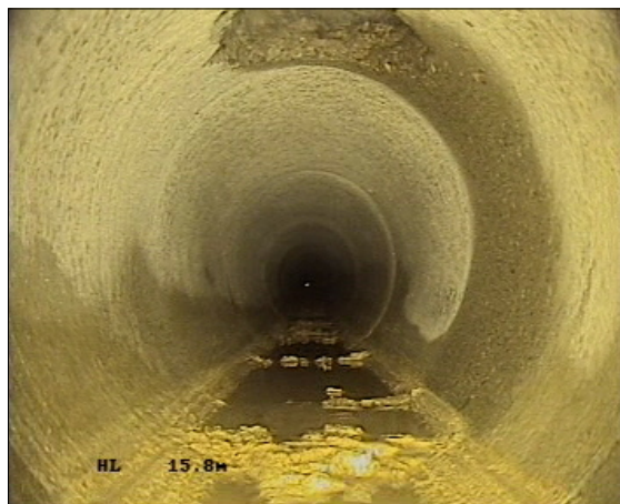
Photo: 8_5A, Media No.: 010208_1, 00:04:20 48FT, Tap Break-In Active, at 12 o'clock, 5", within 8 inches of joint: YES
