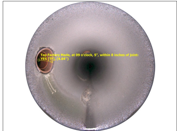
Photo: 7_5B, Media No.: 010208_1 134.91FT, Tap Factory Made, at 09 o'clock, 5", within 8 inches of joint: YES
