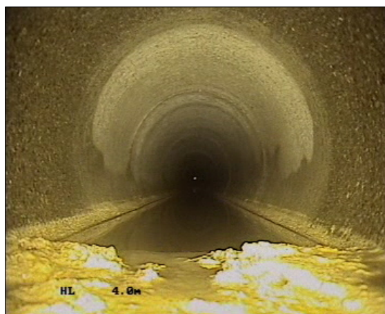
Photo: 8_3A, Media No.: 010208_1, 00:01:26 12FT, Deposits Settled Other, 5 %of cross sectional area, from 05 to 07 o'clock, , within 8 inches of joint: NO
