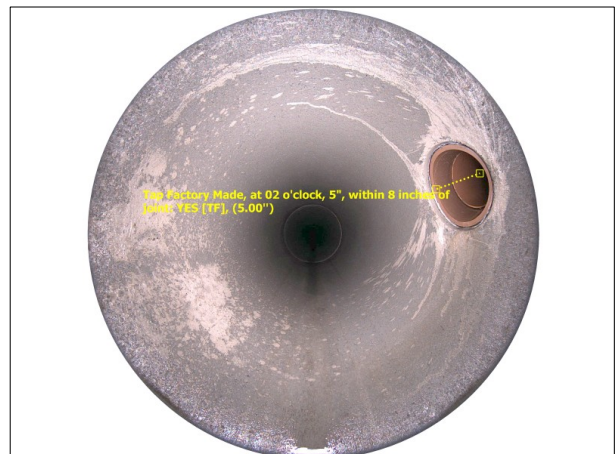
Photo: 7_10B, Media No.: 010208_1 244.04FT, Tap Factory Made, at 02 o'clock, 5", within 8 inches of joint: YES
