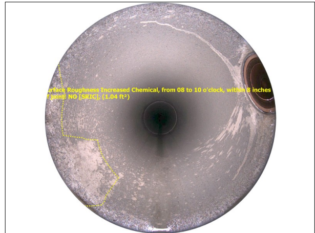
Photo: 7_11B, Media No.: 010208_1 244.14FT, Surface Roughness Increased Chemical, from 08 to 10 o'clock, within 8 inches of joint: NO
