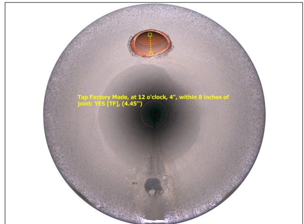
Photo: 7_2B, Media No.: 010208_1 29.73FT, Tap Factory Made, at 12 o'clock, 4", within 8 inches of joint: YES
