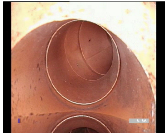
Photo: 4_3B, VCR No.: 010208_1 20FT, Tap Saddle, at 02 o'clock, 5", within 8 inches of joint: NO
