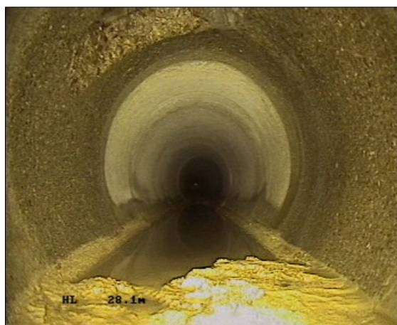
Photo: 8_6A, Media No.: 010208_1, 00:07:46 85.5FT, Tap Break-In Active, at 11 o'clock, 5", within 8 inches of joint: YES
