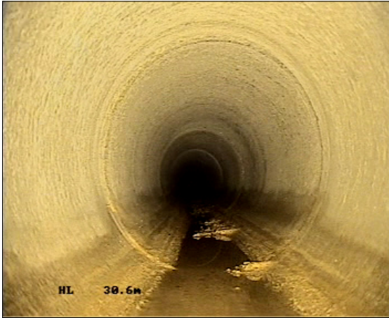
Photo: 8_7A, Media No.: 010208_1, 00:10:20 111.9FT, Deposits Settled Compacted, 5 %of cross sectional area, from 03 to 06 o'clock, , within 8 inches of joint: NO
